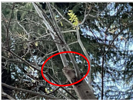
①大枝、樹皮欠損腐朽
