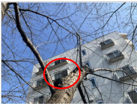
①大枝、樹皮欠損腐朽
